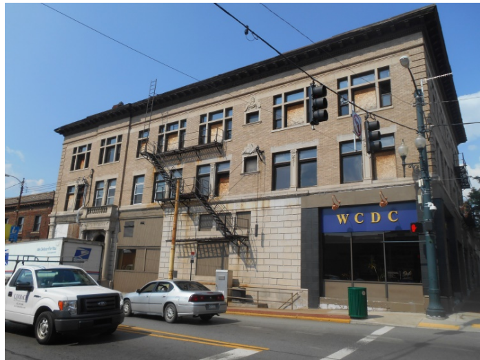
Particle boards in the windows are a clear sign of vacancy/neglect
